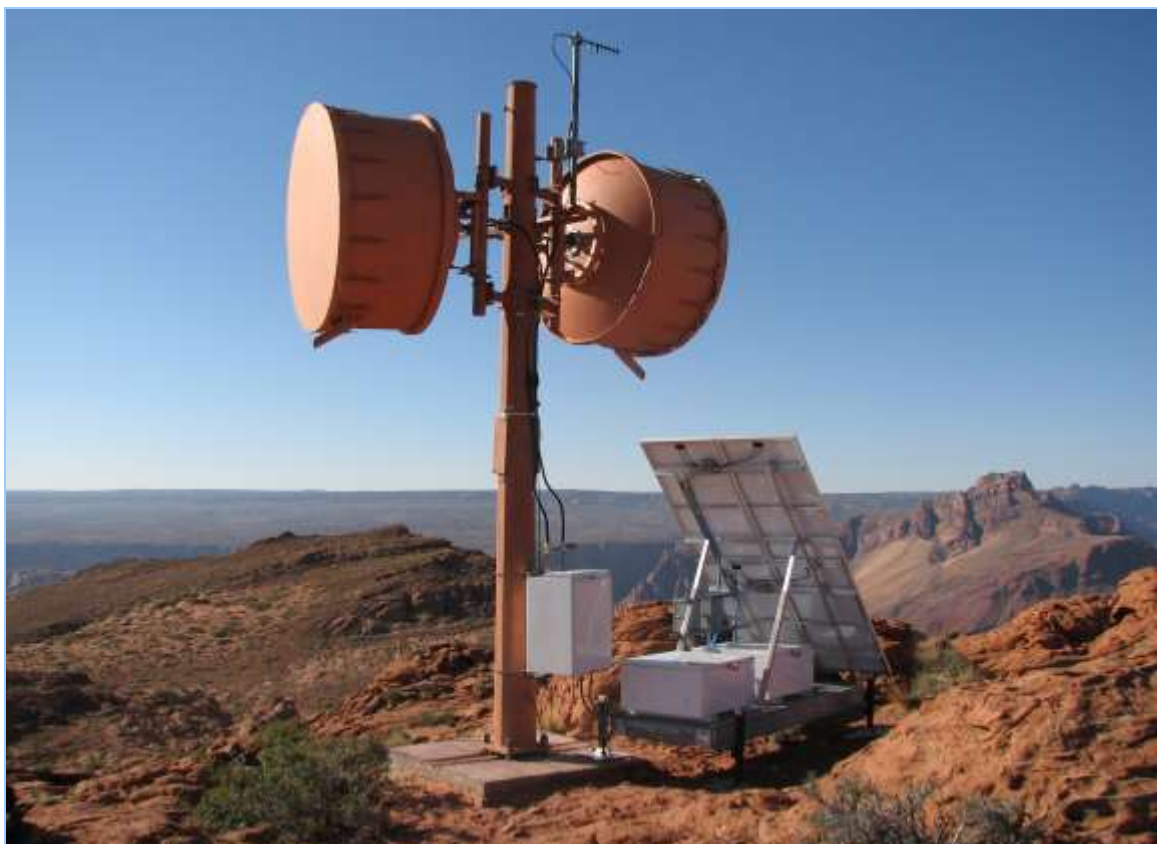
Figure 6 RF Repeater Installation with Solar Power
