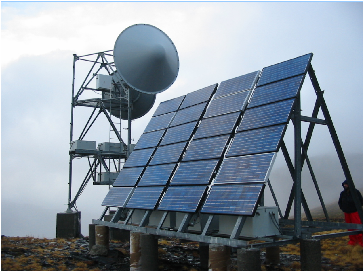
Figure 6 RF-2000E Repeater Installation with Solar Power
