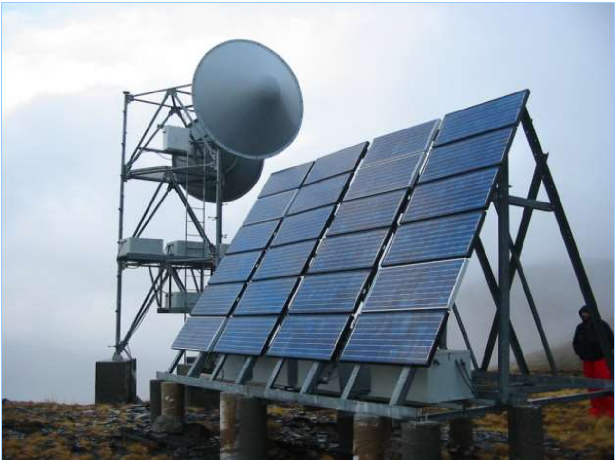
Figure 6 RF-2000E Repeater Installation with Solar Power
