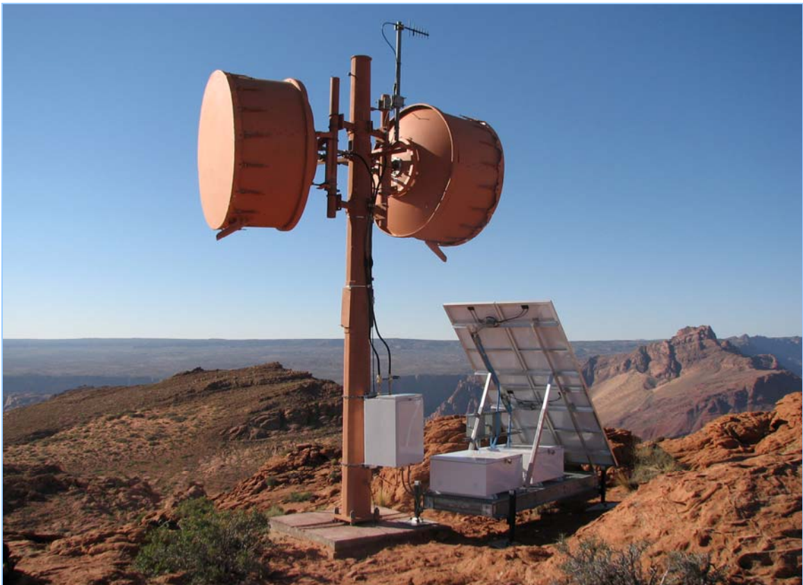
Figure 6 RF-11000 Repeater Installation with Solar Power
