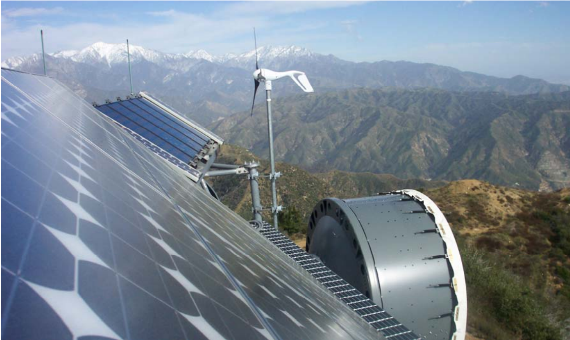
Figure 15 Example of Solar and Wind Power Installation
