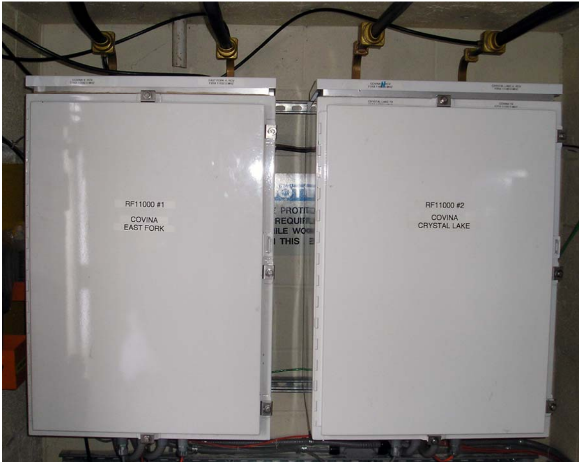
Figure 14 Example of Wall Mounting RF-11000 Repeaters. Note the use of rigid W/G bends and twists.
