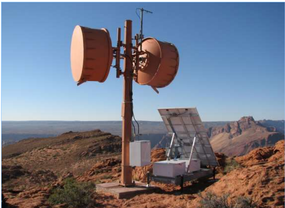
Figure 6 RF-11000 Repeater Installation with Solar Power
