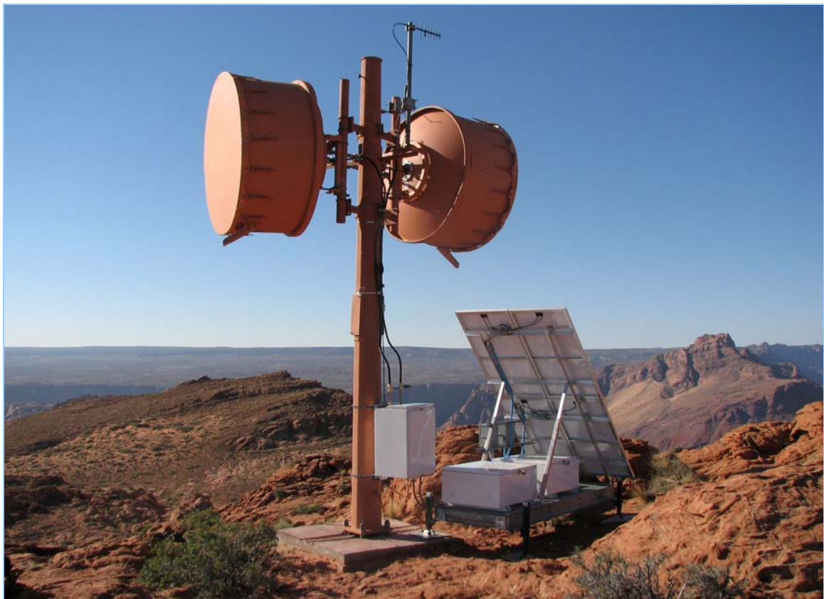
Figure 6 RF-11000E Repeater Installation with Solar Power
